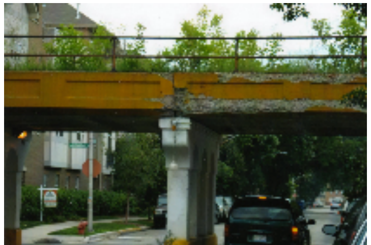
The viaducts are showing a lot of wear and tear
