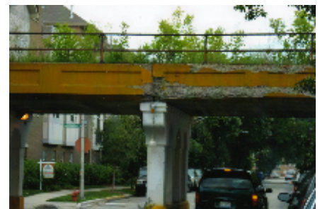
The viaducts are showing a lot of wear and tear.
